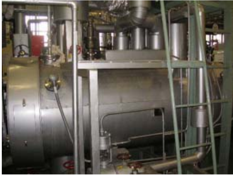
Fig. 2.4.2-1 Pressure Vessel for steam exposure test
